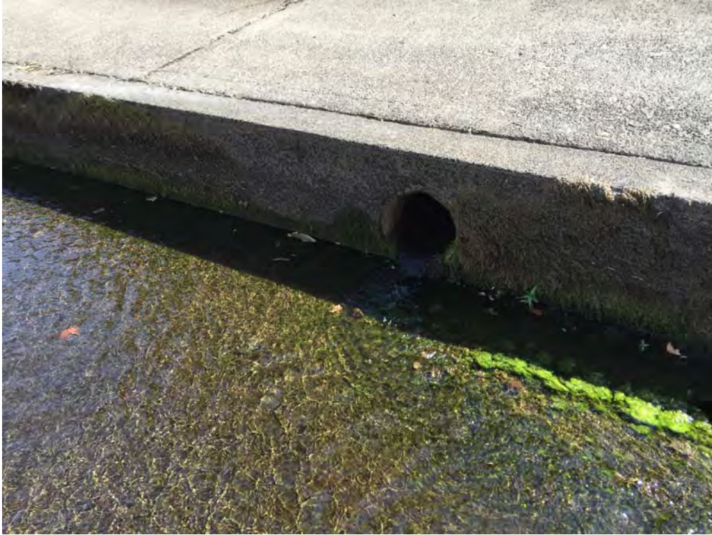
Photo 20 – Spring/Groundwater enters the channel from STA 104+00 to STA 73+00. Flow increases from 0.2 cfs to approximately 2 cfs.
