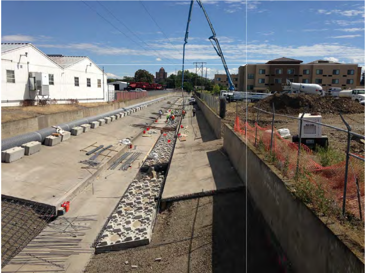
Figure 19 - View from 9 th Avenue of the during construction fish passage elements (baffles, roughness panels, and resting pools). The ramp in the left foreground is the ford to allow county maintenance vehicles to cross the channel.
