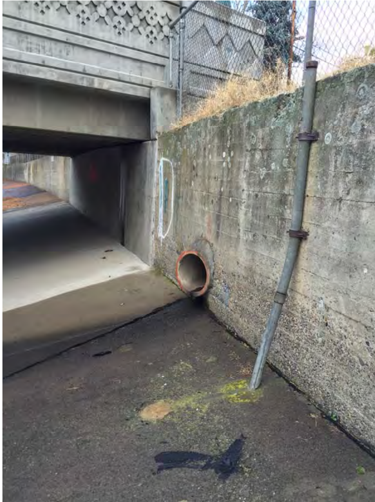
Photo 17 – 2” Galvanized stand pipe and 15” Concrete Drain Pipe.
