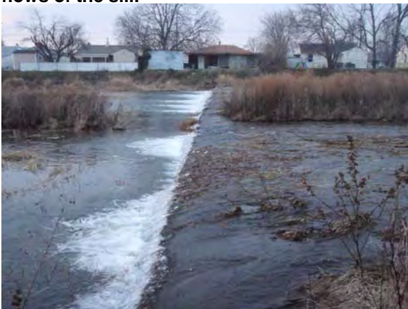
Photo 7-3: Concrete Sill in Segment C RM 9.2 showing vegetation which controls lower flows of the sill.
