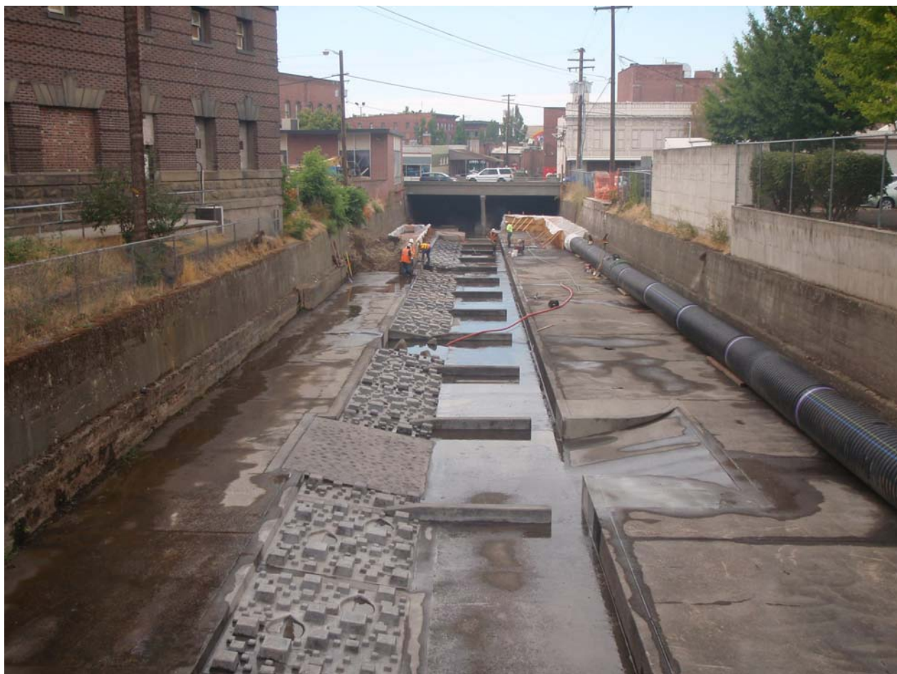
Figure 27 – View from Spokane Street of the completed fish passage elements (baffles, roughness panels and resting pools). The ramp in the foreground was developed as a ford for County maintenance vehicles to cross the channel.
