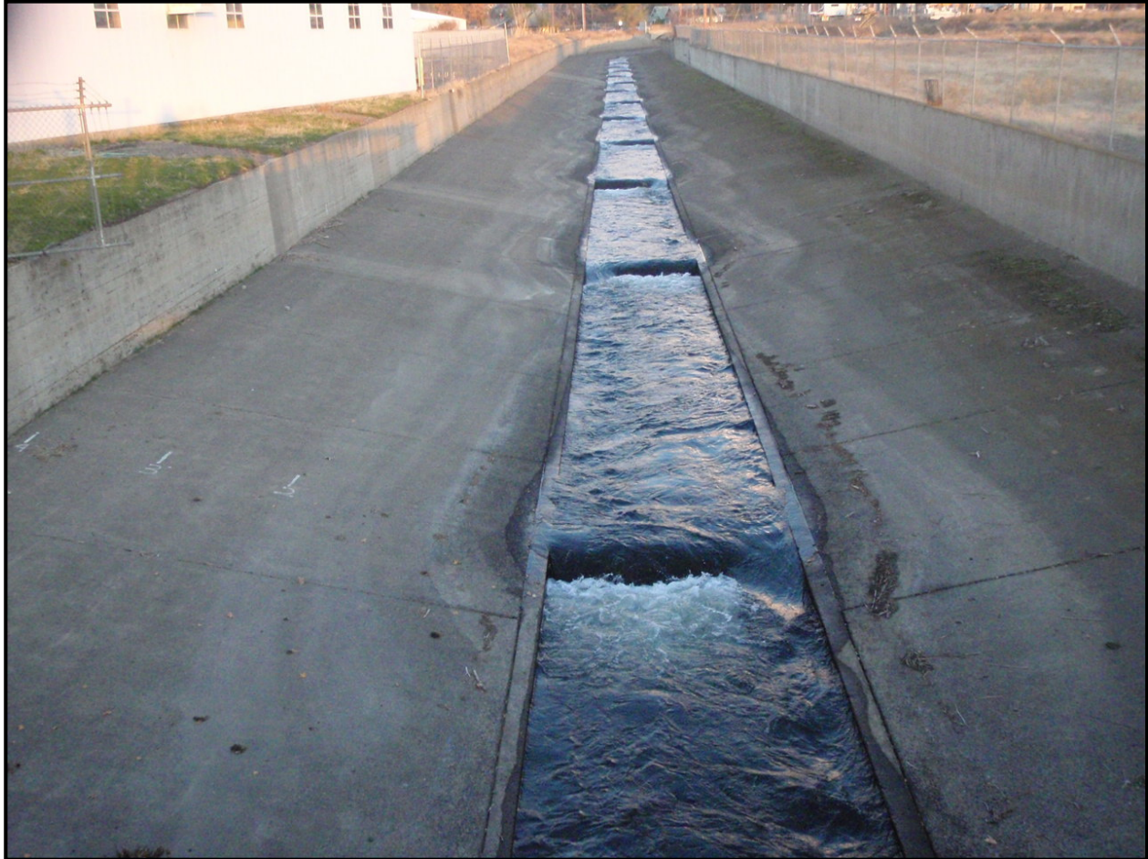
Figure 1 - Upstream view of project area at 25 cfs. The overbank areas are sloped 1:5, which designates this segment as a Reach Type 3 per the Mill Creek Assessment Report.
