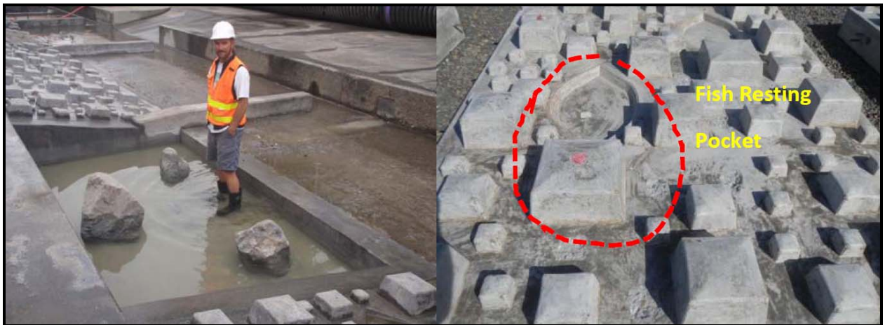
Figure 28 – Photo of Fish Passage Elements: Baffles, Resting Pools and Fish Resting Pockets within Roughness Panels.
