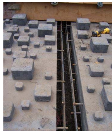
Figure 20 - Panel to Panel Enclosure Curbs 10 inches.
