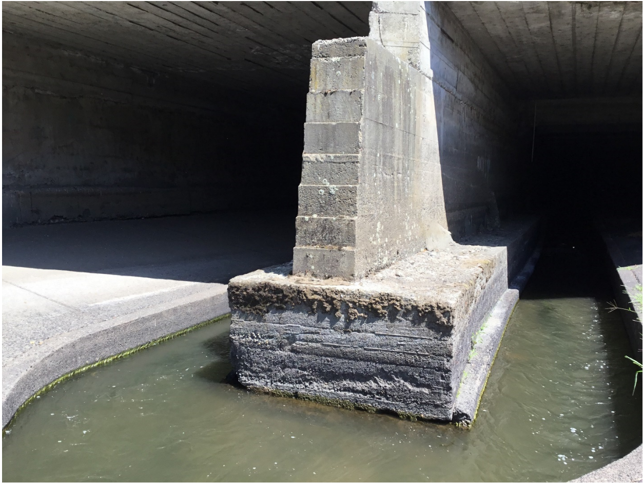
Figure 2 Upstream end of project showing center wall and concrete footings just upstream of end of project and below the 3 rd Avenue Bridge and USCOE Plaza. Looking up stream into the underground section of the Mill Creek. STA 31+06
