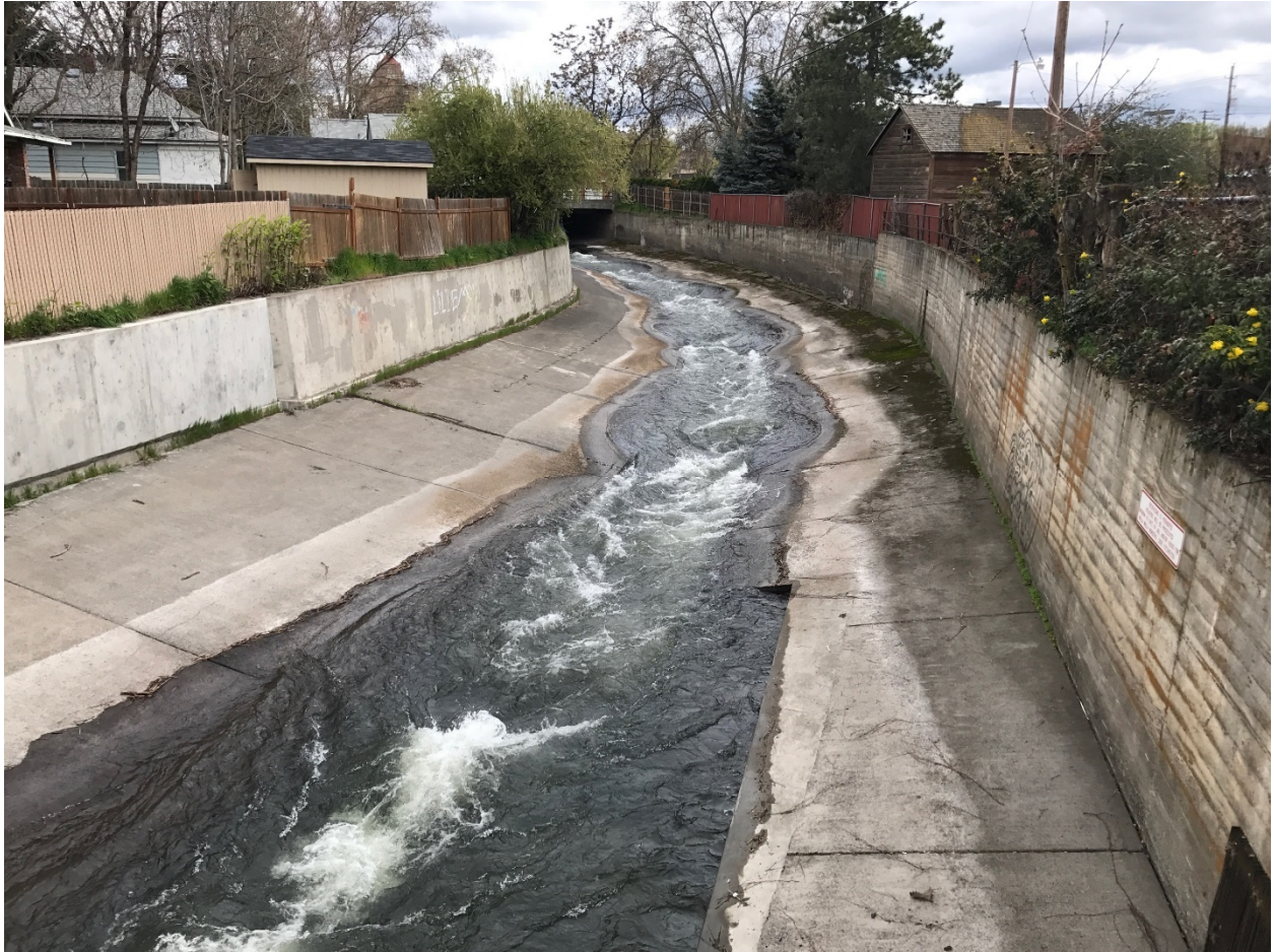
Figure 5 Near the start of project STA 21+25 looking upstream just upstream of the 6th Avenue Bridge. Concrete overlay of the roughness panel for vehicle travel can be seen on the Mill Creek left bank on the lower center of the photo.
