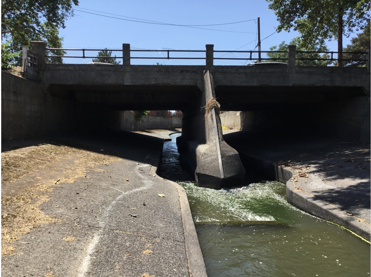
Figure 4 Upstream end of 5th Avenue Bridge and Pier assumed to be removed prior to this proposed reach work. Proposed access site is on the top left side of this photo.
