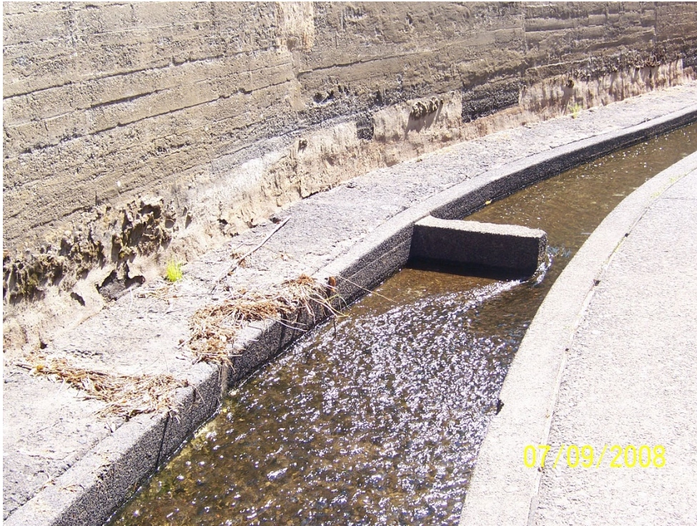
Photo 3 – View upstream in Reach Type 7 with flat overbank showing 4.5-foot-wide trench and 3.5-foot-long baffle.
