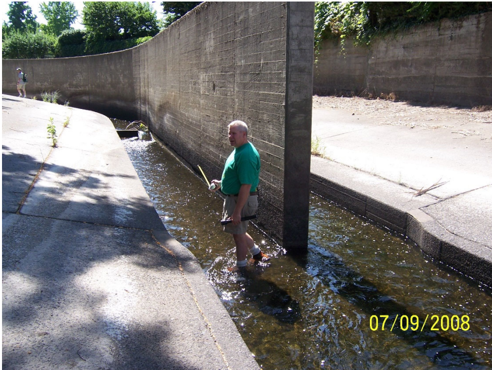
Photo 4 – View upstream of Reach Type 7 center wall with sloping overbanks and Engineer Jay Kidder of Chinook Engineering.
