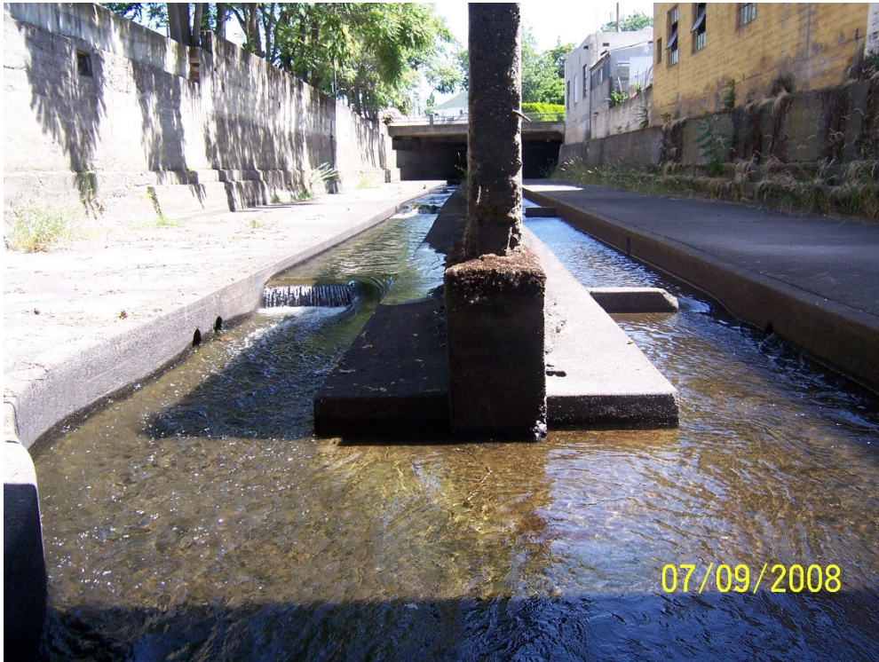
Photo 1 – Downstream end of project showing center wall and concrete footings just upstream of Spokane Street.
